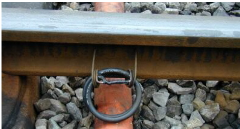
Figure 8 - "D Link" termination
