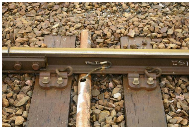
Figure 4 - Cable Secured in Orange Pipe
